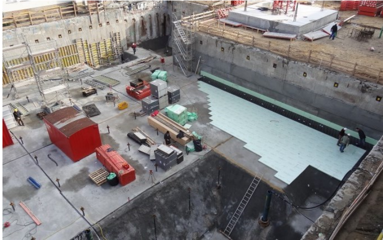
Construction activity in the rear building section in 2016. Deepest point: 13-meter excavation for the foundation of the NION-TEM.
